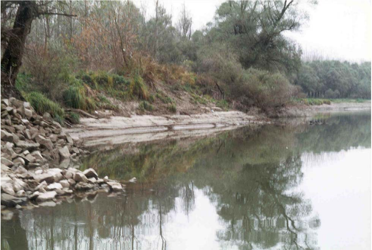
Photograph 6. The left bank of the Vén-Duna at the reopened rock dam at low water level
